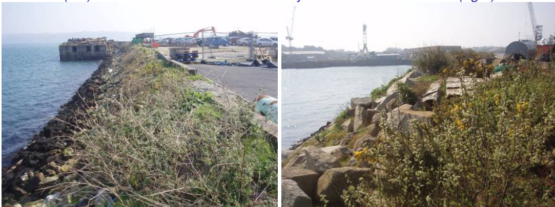
Figure 10-1 Vegetated Rock Revetment between Queens Wharf and Northern Wharf (left) and Willow and Gorse Scrub adjacent to Northern Wharf (right)
