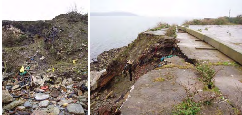
Figure 2-7 Coastal Erosion along the Existing Waste Tip in the Eastern Docks
