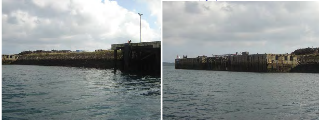
Figure 2-4 Existing Area between the Northern Wharf and Queens Wharf (left) and the Existing Northern Wharf (right)
